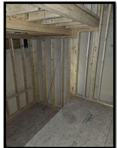
Room is two-levels to accommodate the airflow
